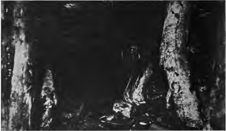
Fig. 14. Broken Timber in Room, Pioneer Iron Mine, Oliver Iron Mining Co., Ely, Minn.
